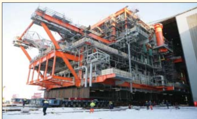
The 11,000-ton Valhall redevelopment integrated production and hotel facility deck, being built for BP Norge, leaves the fabrication hall at Heerema Zwijndrecht, one of the three production locations of Heerema Fabrication Group. Photo from HFG.
